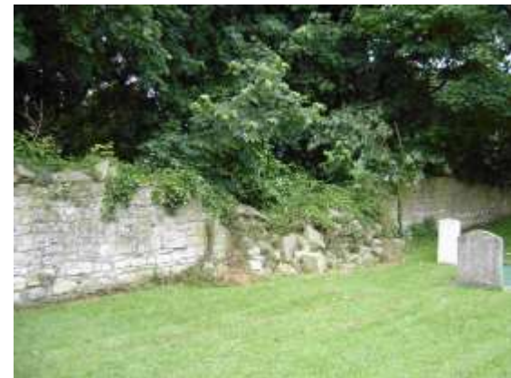
Part of the wall that has fallen down.
