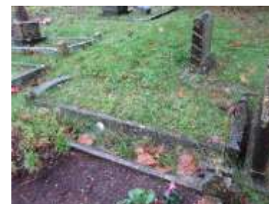
Edging. The leaded inscription is on the upper surface. The northern part of edging has fallen down.
